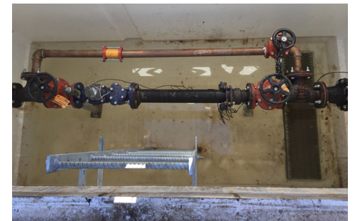
Newly installed large water meter
